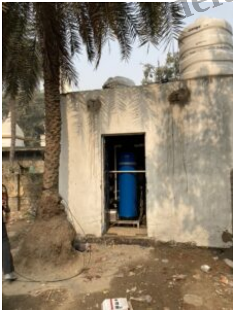
RO unit and building
