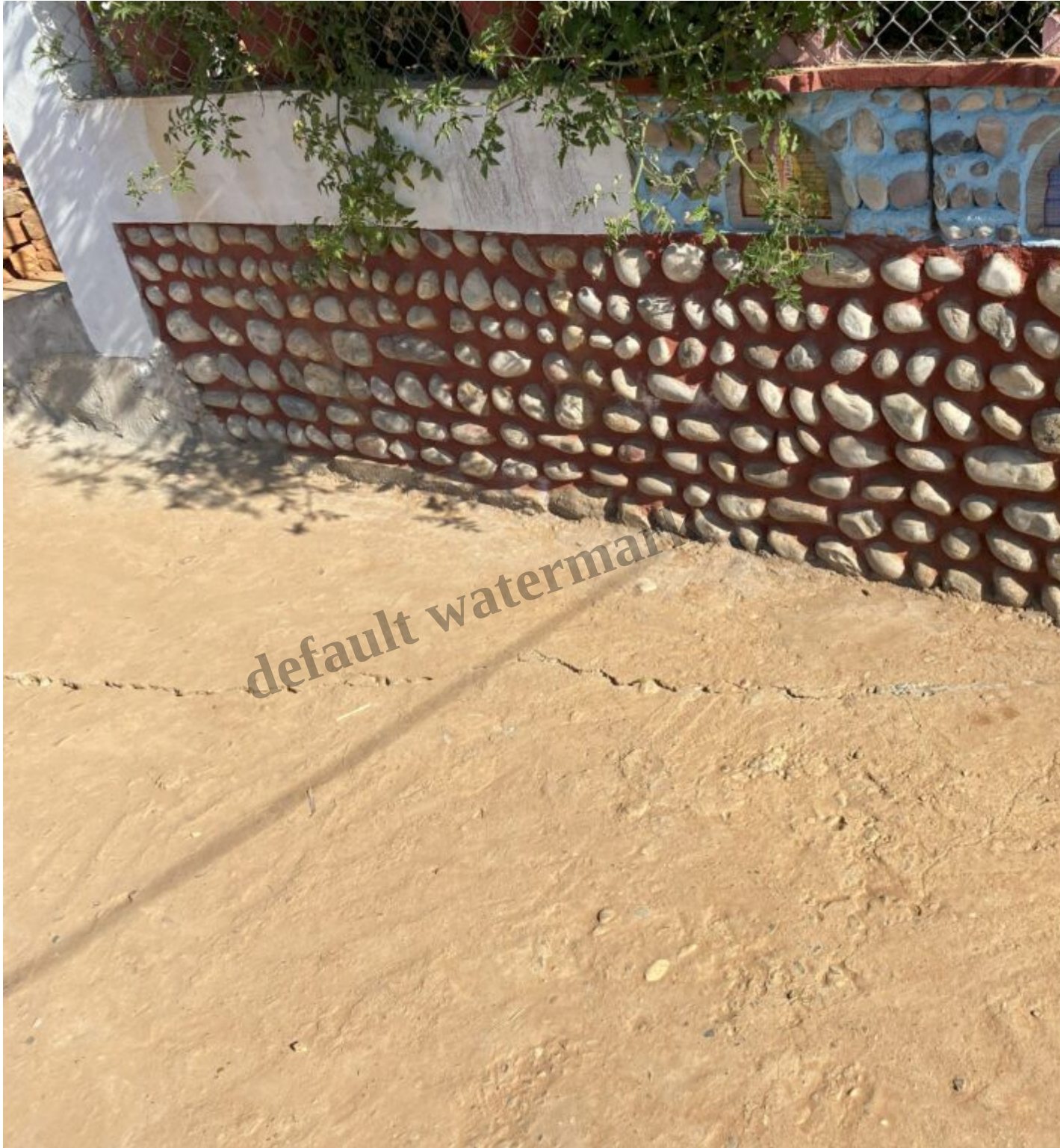
Crack in the road
