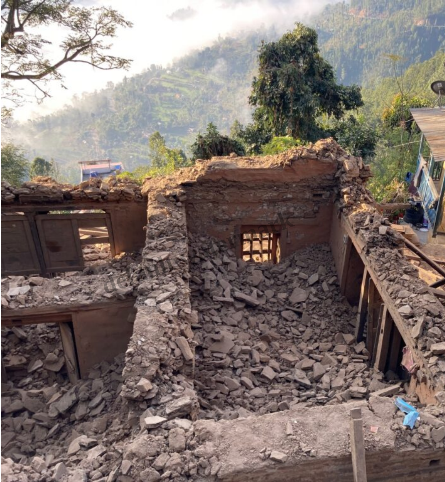
Destroyed next to Intact
